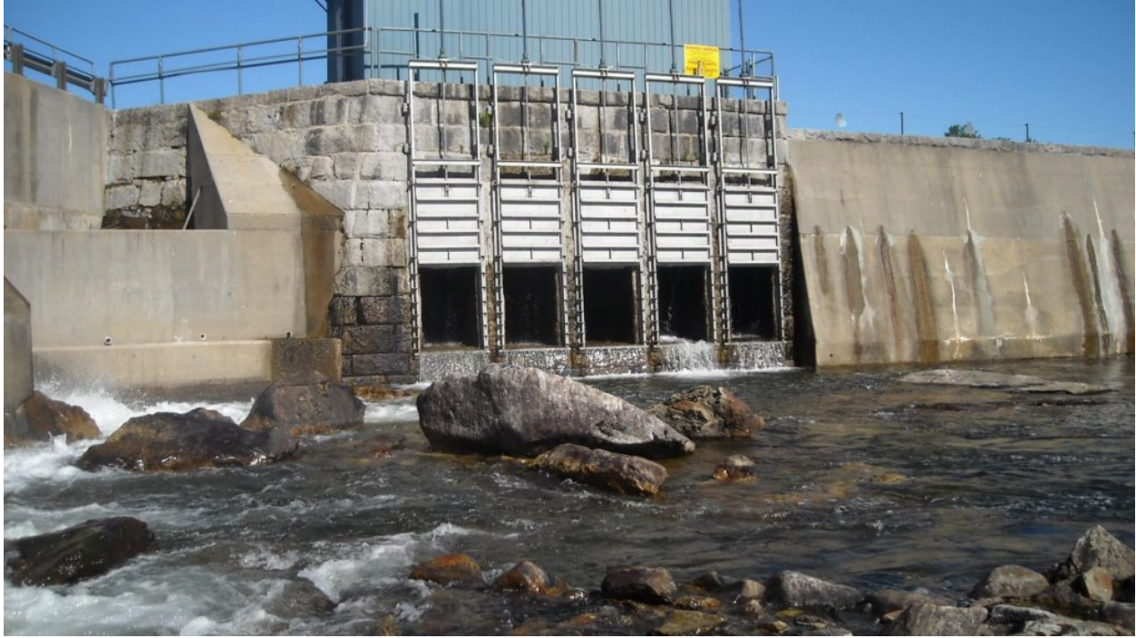
Pictured is the Eel Weir Dam powerhouse, the building thereof at the head of Sebago Lake caused a host of cascading effects. PHOTOGRAPH BY ROGER WHEELER
